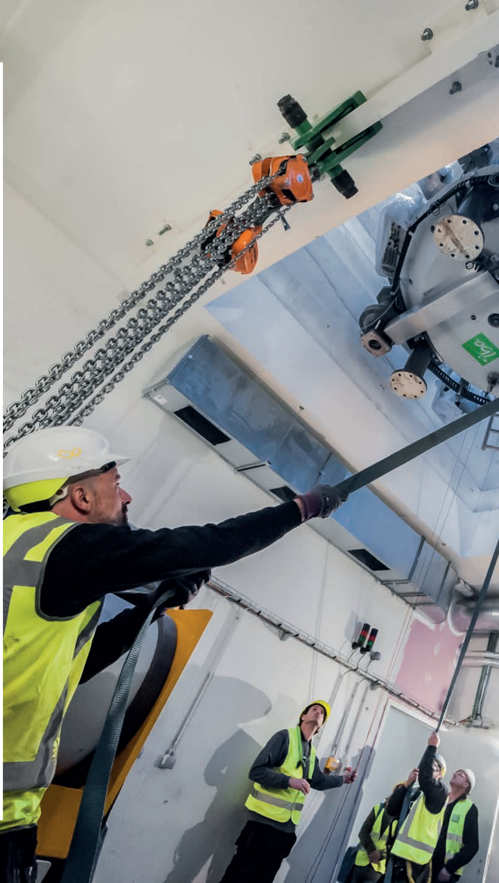
Installation of an IBA cyclotron at Belgium's first proton therapy center at the hospital in Leuven, Belgium, 2019.
